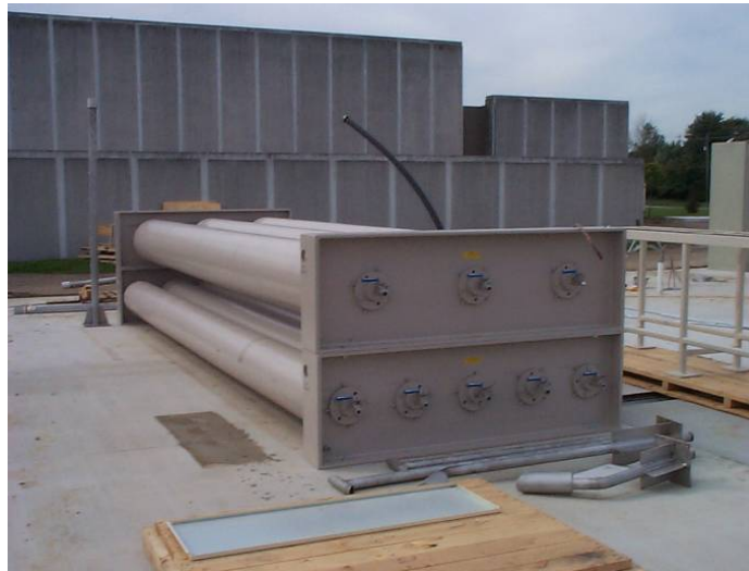
Figure 5. High-pressure hydrogen or CNG storage tanks
